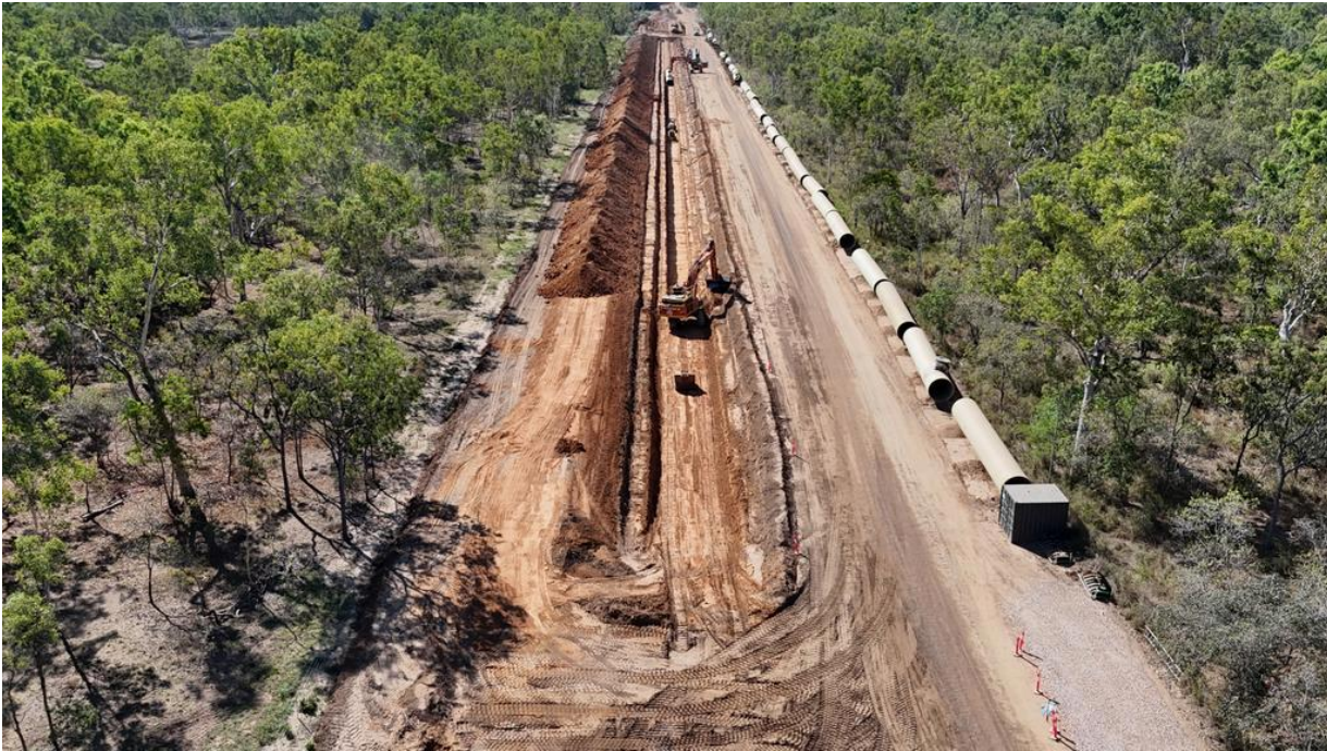
Glass reinforced polymer pipes being laid south of Townsville for stage two of the Haughton Pipeline. Picture: Supplied.
