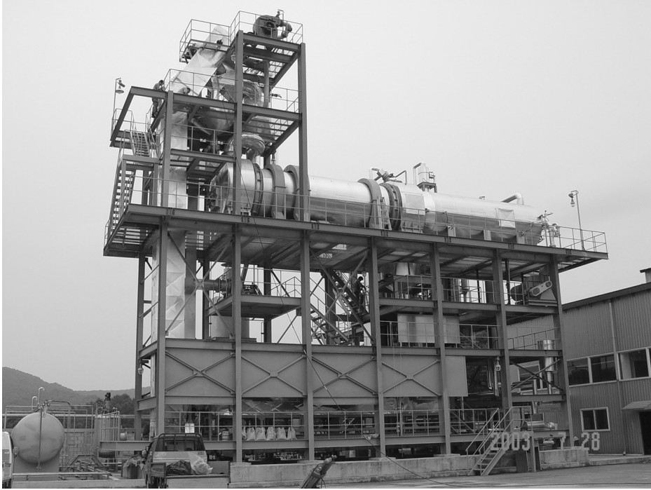
Figure 15.14 Photograph of the Reentech catalytic cracking process in Korea. The Reentech process converts mixed plastics (e.g. PE, PP, PS) into gasoline, kerosene and diesel fuel. (Courtesy of Reentech, Korea)
