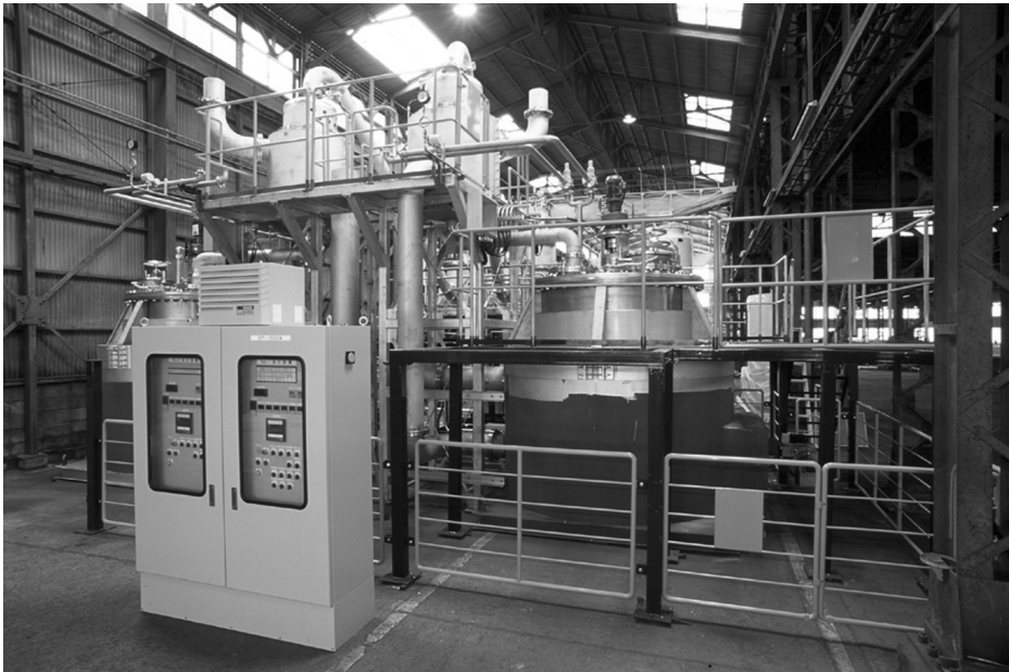
Figure 15.9 A commercial Thermofuel™ plant in Okinawa in Japan which processes agricultural plastics such as mulch and greenhouse films into diesel fuel to run greenhouse boilers for heating, tractors and other agricultural machinery. (Reproduced by permission of Ozmotech Pty Ltd)
