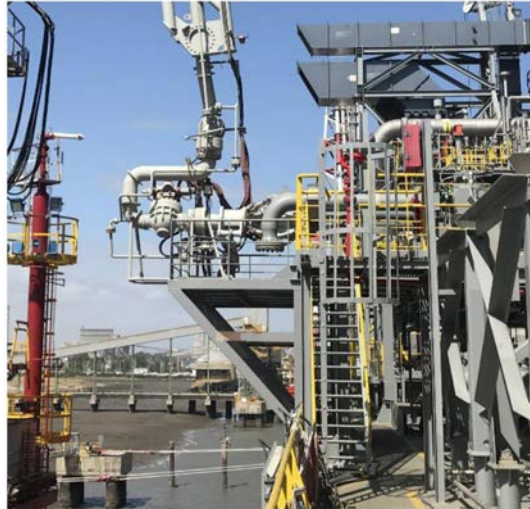
Figure 13—HP loading arm connection
