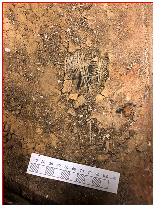
Fig. 4. Top of GCL showing partly degraded upper cover GTX around and over a bentonite hole 40 mm long and 20 mm wide.
