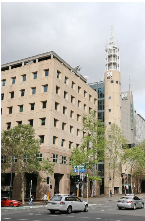
Figure 3 It is expected the cladding will be removed next year. Picture: Richard Dobson
