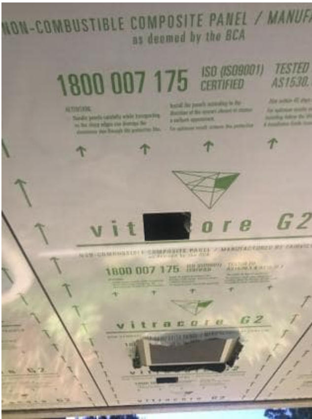
Figure 2 New non-combustible cladding being installed at Oatley station in August 2018. Picture: Supplied
