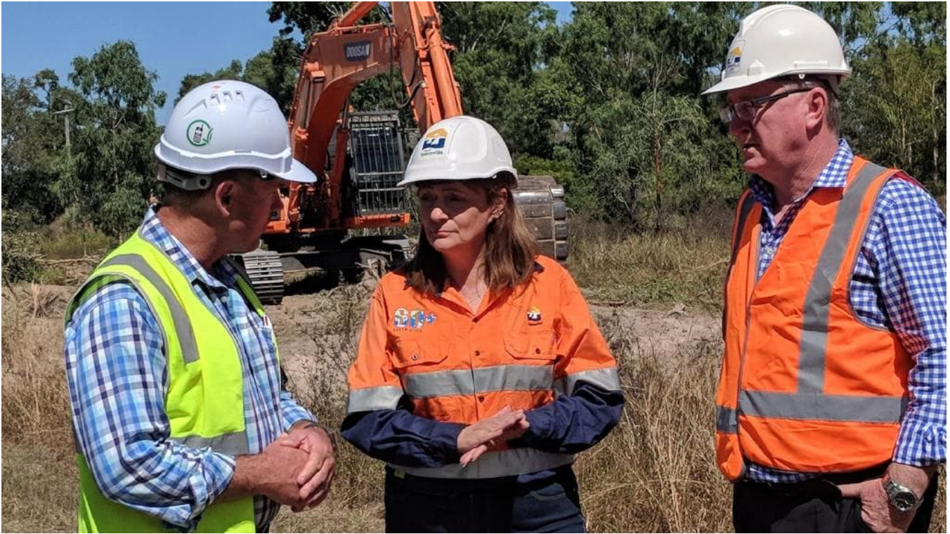
Figure 2 Mendi Group managing director Jeff Doyle with Mayor Jenny Hill and Deputy Mayor Les Walker marking the start of civil work on the Haughton water pipeline project.
