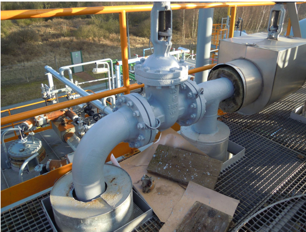
PPG HI TEMP 1027 was used to protect pipes and valves against CUI in severe cyclic temperature service.
