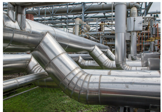
Picture 1: Insulated high temperature piping
