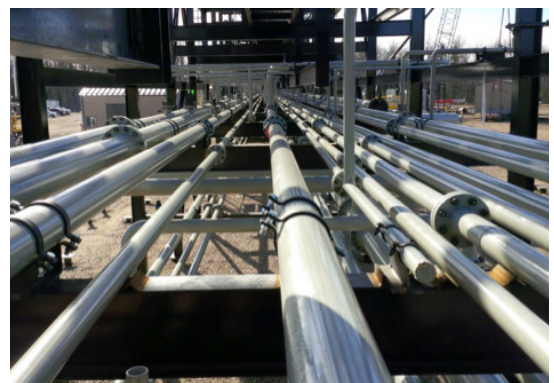
Picture 2: Uninsulated high temperature piping
