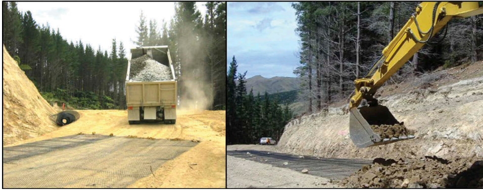
Figure 7. Covering geogrid with aggregate can be achieved with a dump truck (left) or excavator (right). Note that the maximum rock size in this aggregate is too large and can easily cut the geogrid.
