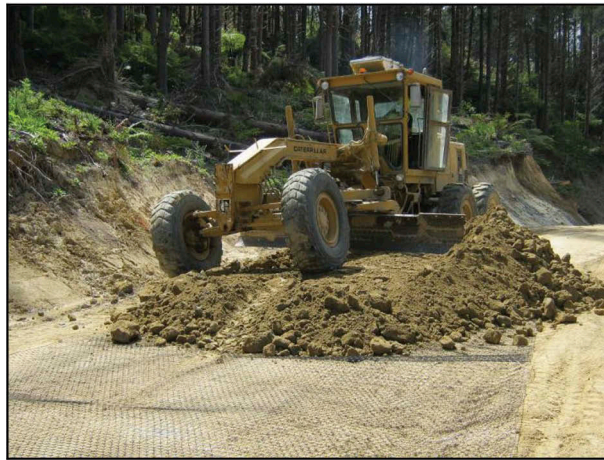
Figure 8. A grader being used to spread aggregate over geogrid. Note that it is very difficult to judge aggregate depth using this technique.
