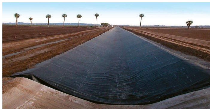
Fig. 6. GCL Placement as a Canal Liner in an Irrigation Canal (Geosynthetic Materials Association, 2010)
