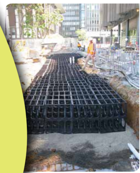
Terravault installed at Monash Transport Interchange, ready to be filled with soil
