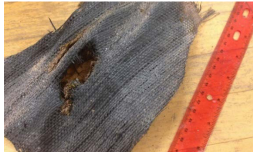
Figure 9. Large hole in the geotextile due to improper geotextile installation
