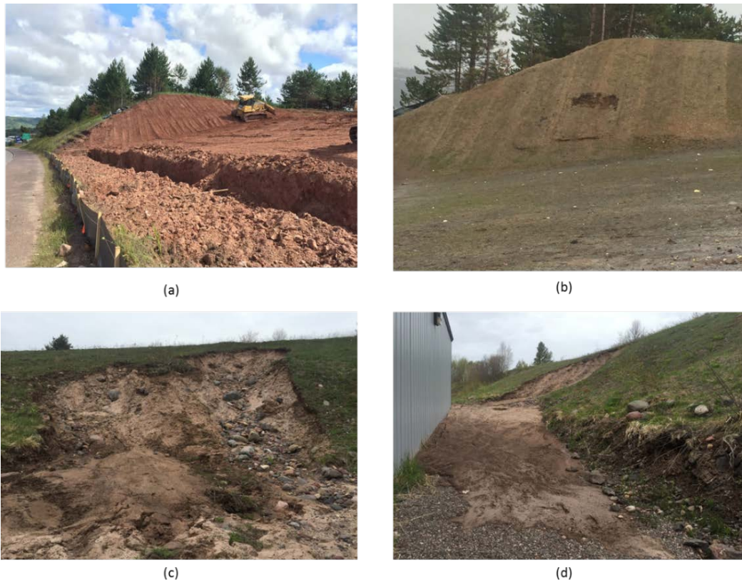
Figure 2. Spring, 2016 small scale landslides in the Hancock-Houghton area: (a) slope constructed in fall 2015 and sodded, (b) spring 2016 small scale failure on slope; (c) small landslide on an established slope, (d) soil flowing behind a commercial building.
