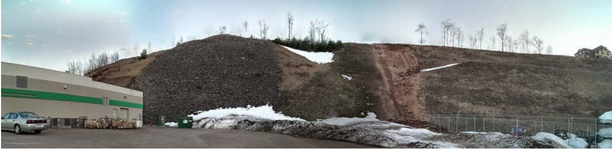
Figure 3: Commercial site with excavated slopes in the range of 30° to 40° that experienced three slope failures. The middle section of the slope, which failed first, was remediated with rock rip-rap, while the slope failures on either side have not been remediated
