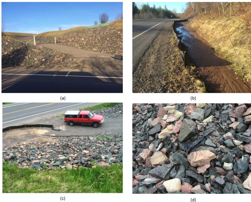
Figure 5. Road accessing M-203 with springtime failure: (a) road after the first failure and remediation, (b) silt fence containing additional sand and water still flowing from the slope, (c) 2014 second failure after remediation, (d) geotextile directly under the rip-rap on the slope.
