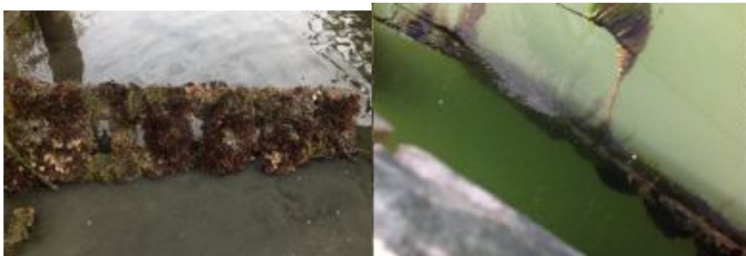
Figure 9. Rig with Marine Growth on December 30 th , 2013 (Winter)
