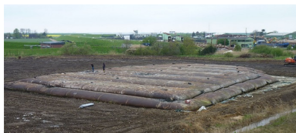
Figure 4 View from the South to the North of the first dewatering field six months after end of operation (note the preparation of the dewatering area for the following main section around the previously used tubes)
