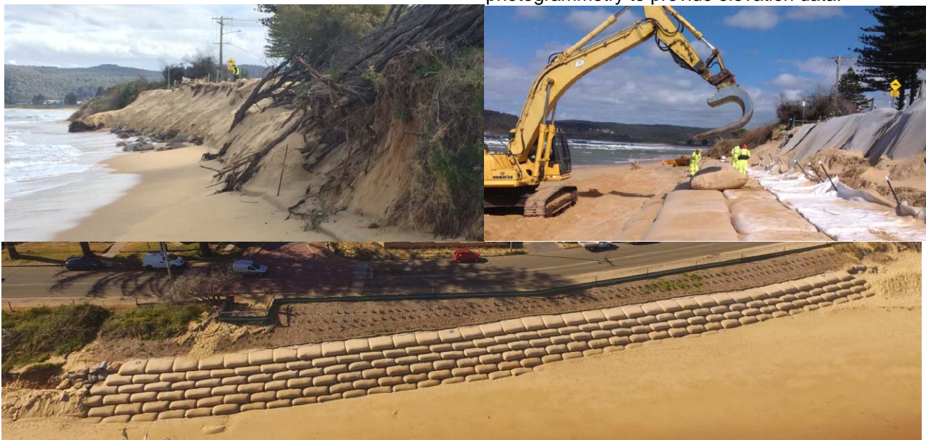
Figure 4 Construction of the GSC seawall. Clockwise from top left: the erosion scarp in August 2015; placement of 2.5 m 3 containers using modified rock grab; aerial view of completed GSC seawall after 3 months in operation.
