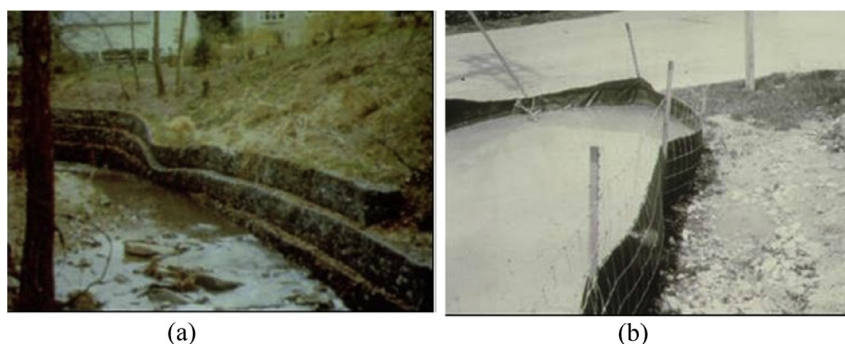
Fig. 2. Improper and proper use of woven silt film fabrics (GSI photos). (a) Gabion wall failure, (b) Silt fence success.
