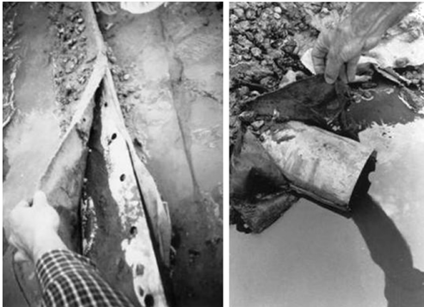
Fig. 4. Geotextile wrapped perforated pipe failure (GSI photos).
